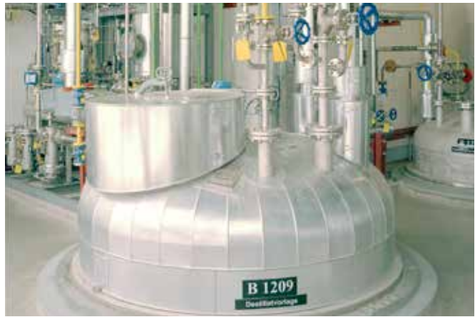
Interior view of Clariant's Licocene production plant Innenansicht der Clariant Licocene Produktionsanlage
